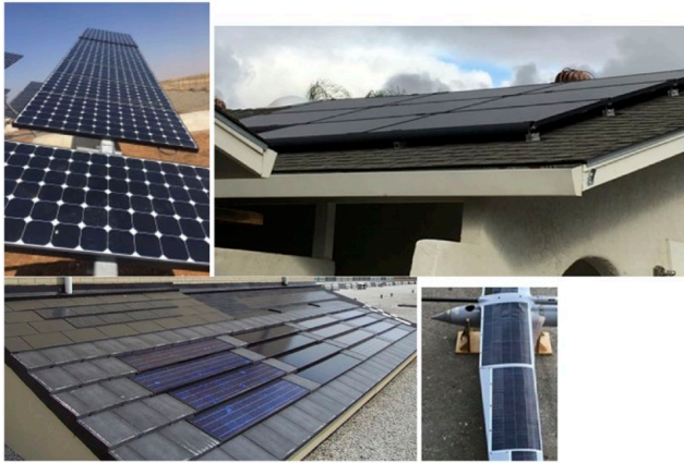
Figure 1. Examples of types of PV systems. (a, upper left) Ground-mounted. (b, upper right) Building-applied (BAPV) in which the PV system is applied to the completed building. (c, lower left) Building-integrated (BIPV) in which one or more building elements are replaced by the solar system (in this example, the solar panels are similar to BAPV panels, but have been mounted in such a way that on the area covered by them, the shingles are not needed), and (d, lower right) surface-integrated system in which thin PV devices are built directly into the surface.
