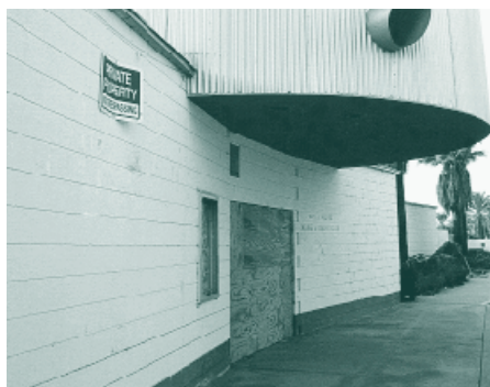
North Shore Yacht Club, Architect Albert Frey. Boarded up structure.
