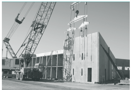
photos: Prison cells under construction at the $750 million Delano II State Prison in the Central Valley. Is this the future for California's next generation?
