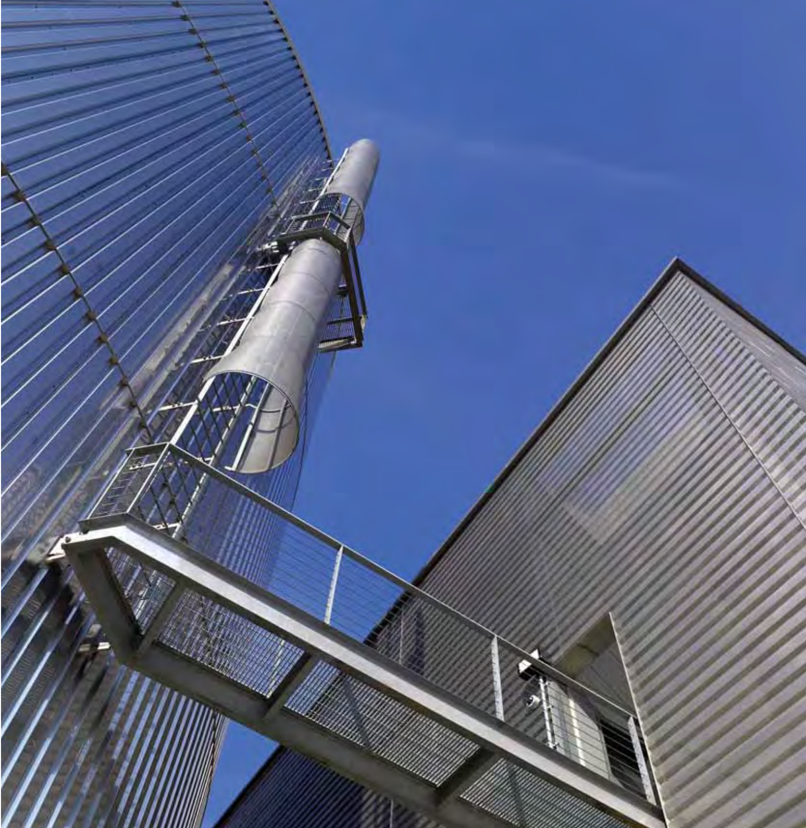
above: UC Merced Central Plant, Skidmore, Owings & Merrill, LLP, photography by Tim Griffith.
